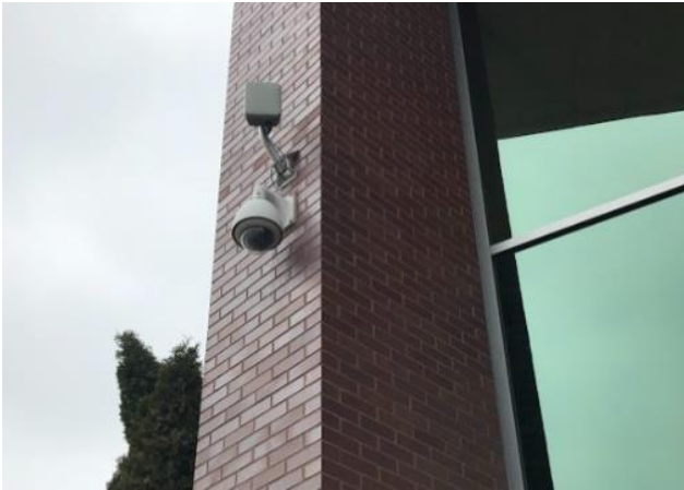
One of 21 existing WiFi access points at Novi Public Library
