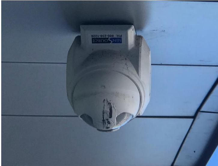
The Car Counter sensor before being hit
